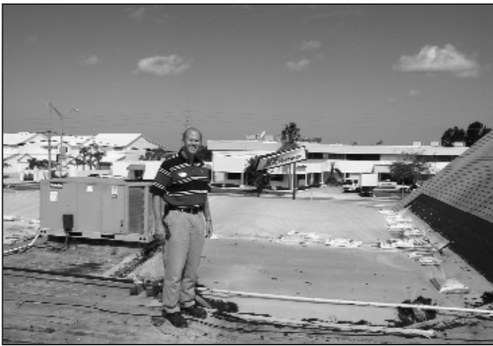
Bill Pastermack shows where the roof of his store in Titusville was damaged. He stayed open by placing plastic over the damage.
