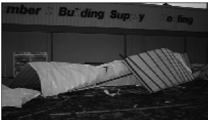
The metal roof of Nicholson's Ace Hardware in rural Wauchula, Fla., blew off and landed in the store parking lot after a direct hit from Hurricane Charley. The store also suffered extensive water damage.
