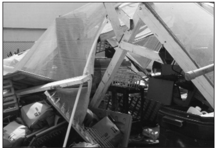
The roof of Ed Struttman's store in Indialantic collapsed and the inside suffered extensive structural damage.
